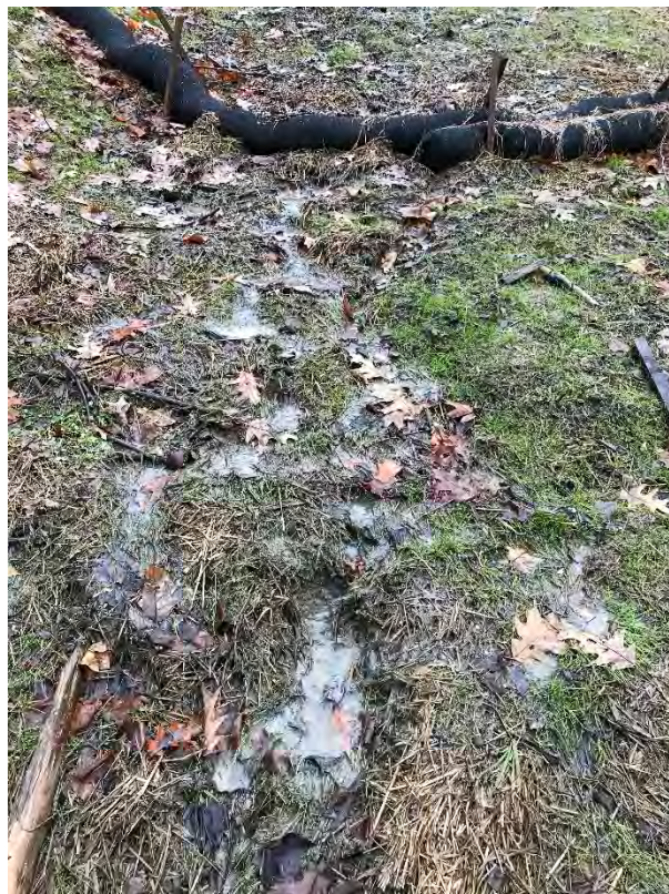
Fig 8: Minor rill and preferential flow path development on lower portion of slope between Strs. 28 and 29. Viewing south. (01-16-21)
