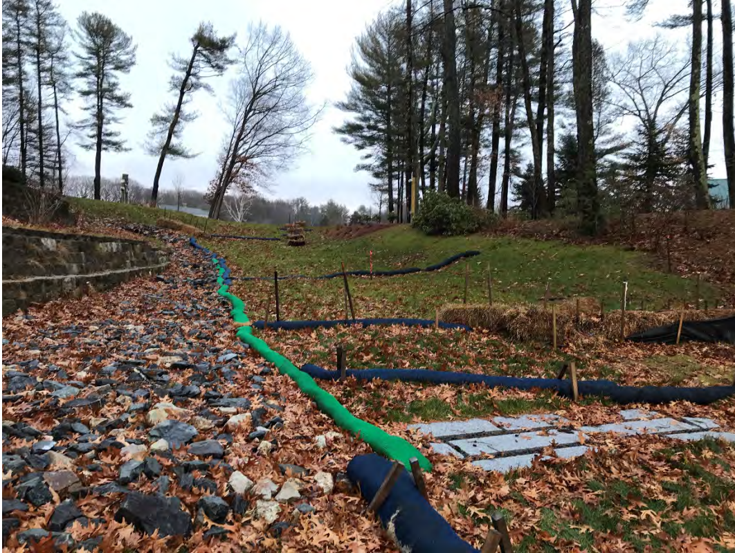
Fig 9: Slope above the manhole at Gundalow Landing/east side of the bay. Viewing east. (01-16-21)
